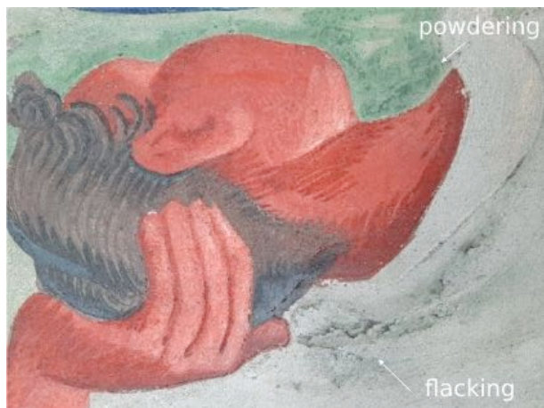
Fig1: Detail of the deteriorated green paint layers found in P5. Maritime Station of Alcântara, Lisbon. Photo by: MGi2021
